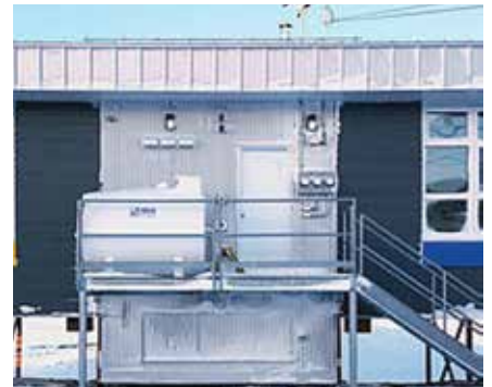
Figure 8: Furnace-oil heating equipment
