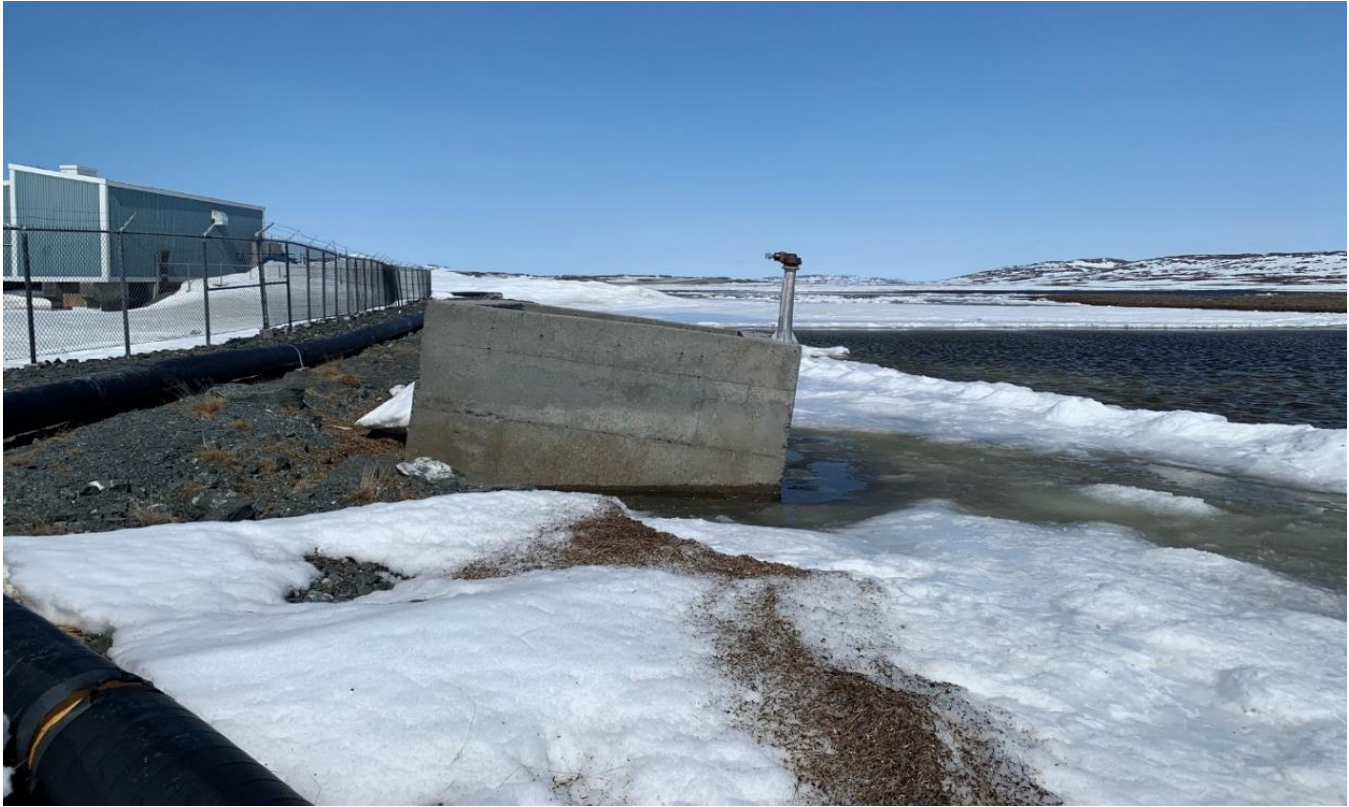
Figure 3. Protective caisson for the water intake pipe on the bank of the Illukotat River. Photo taken on May 19, 2024.
