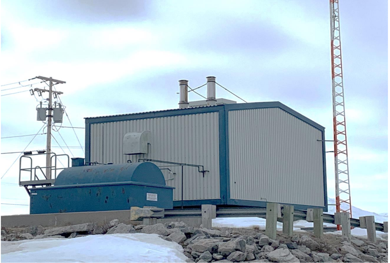
Figure 5. Inukjuak pumping station with diesel tank. Photo taken on May 16, 2024
