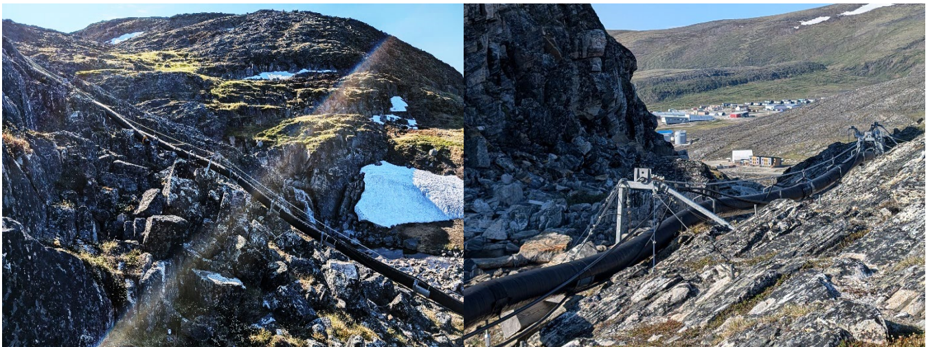
Figure 5. Above-ground positioning of the supply conduit between the withdrawal site and the WTP (Photos taken on July 26, 2024, by Antoine Thibault)
