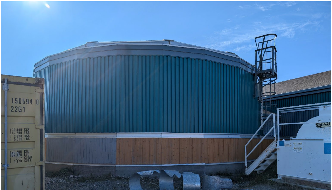
Figure 7. Treated water tank attached to the Kangiqsujaq WTP ( 450 \text{ m}^3 ). Photo taken on July 26, 2024, by Antoine Thibault.
