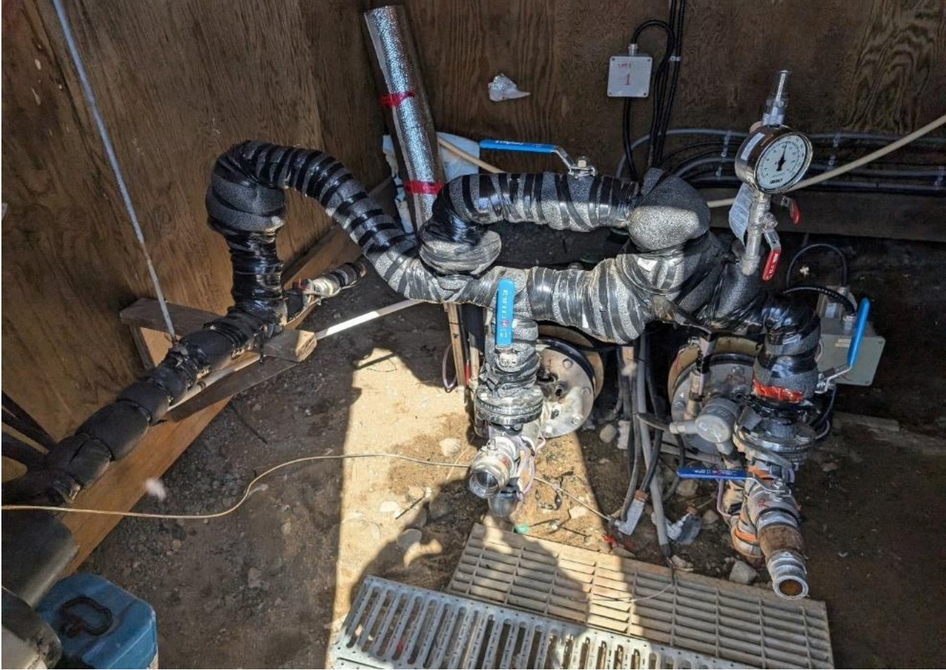
Figure 5. Inside the navy blue building: raw water pumping station (Photo taken on July 7, 2024, by Antoine Thibault)
