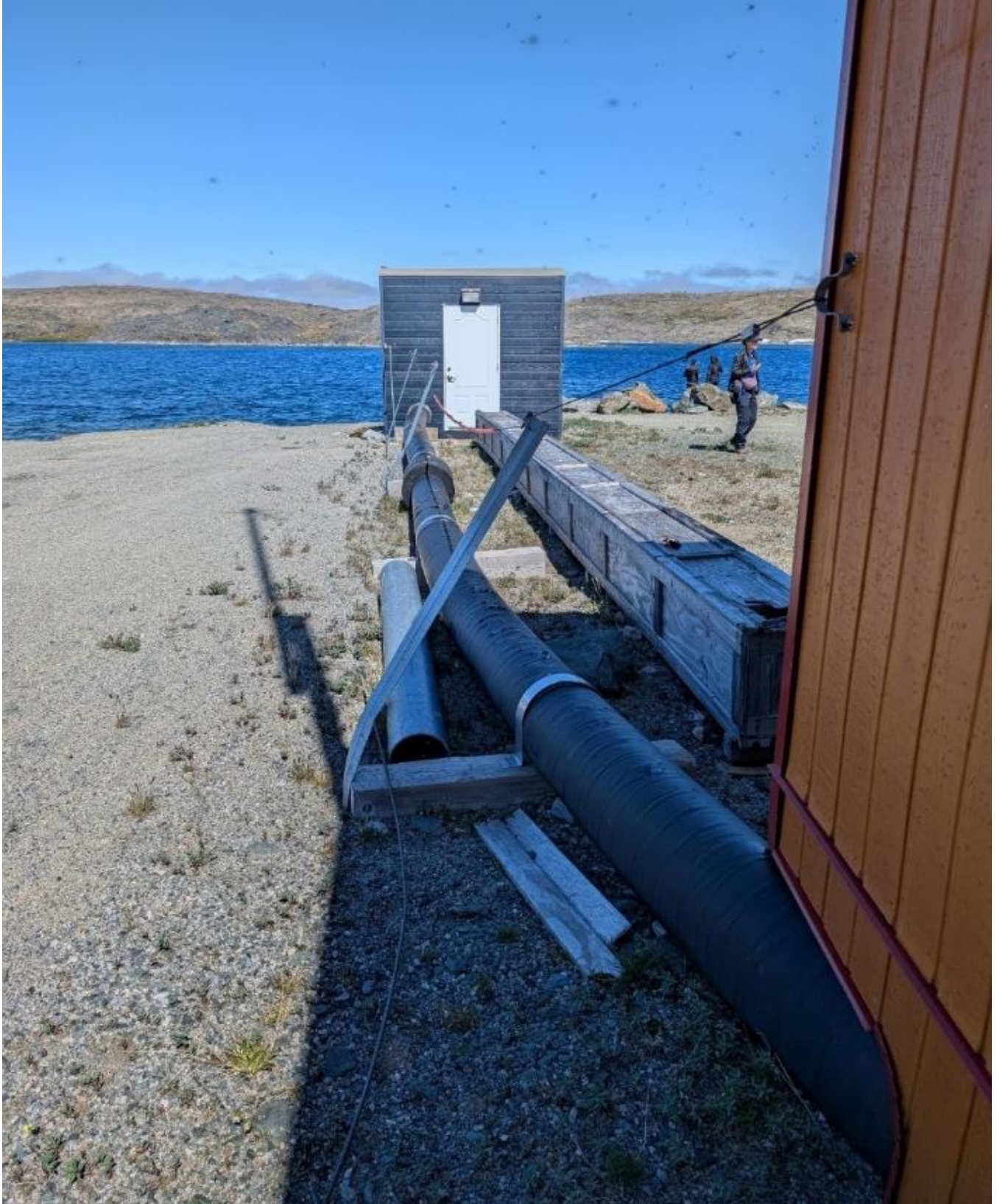
Figure 4. Connection between the building housing the pumps and the pumping station. Photo taken on July 7, 2024 by Antoine Thibault
